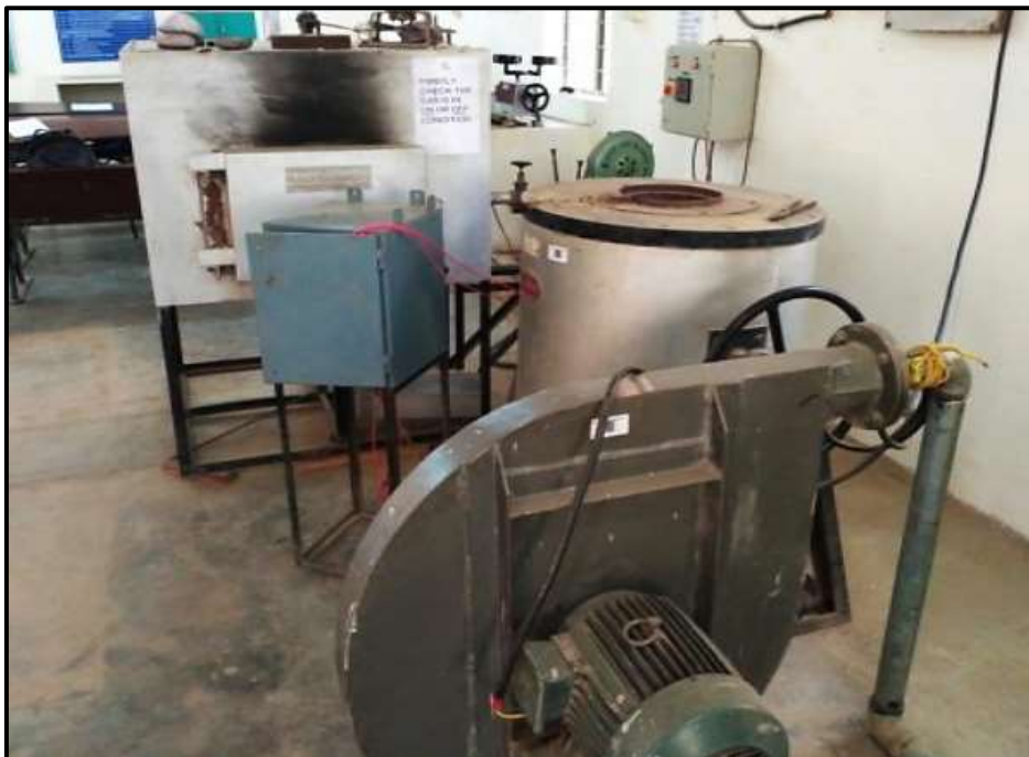
LPG Fired Gas Furnace in Foundry, Forging and Welding Lab
